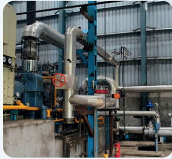
Waste Heat Boilers
