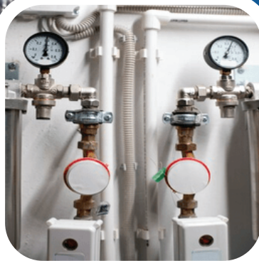
• Pressure Reducing Station
